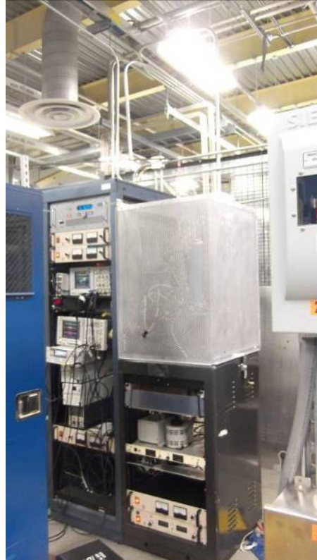
Fig. 22. Test stand for electron beam testing (front and right side). The high voltage parts are closed by metallic mesh shielding.
